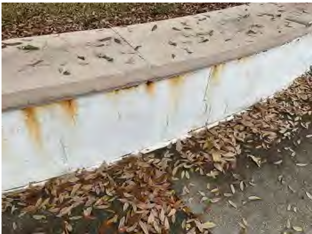
Cracks and rust stains
