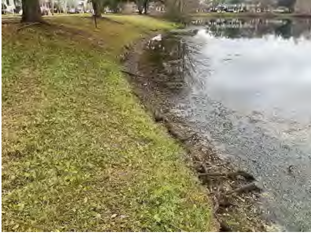
Minor shoreline erosion
