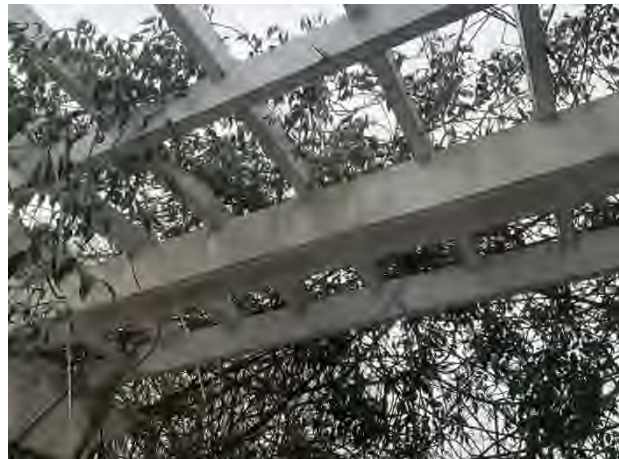
Pergola wood deterioration
