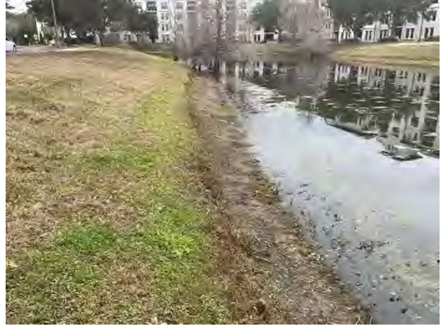
Minor shoreline erosion
