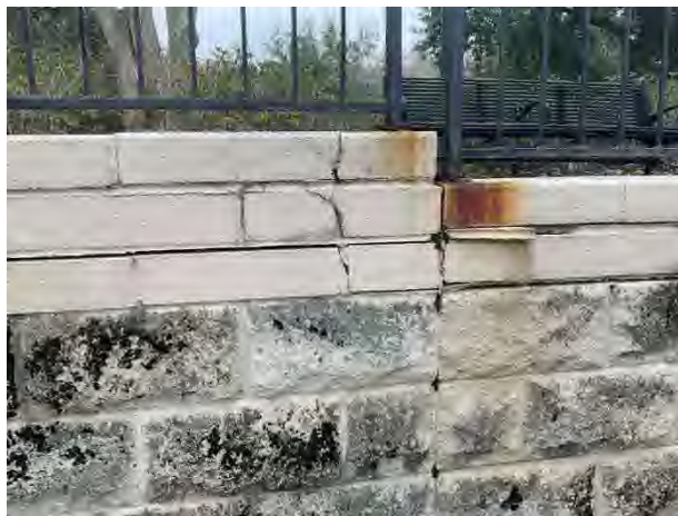
Cracks and settled masonry
