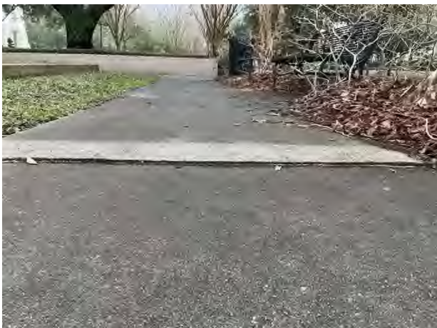
Trap hazard with previous grinding evident
